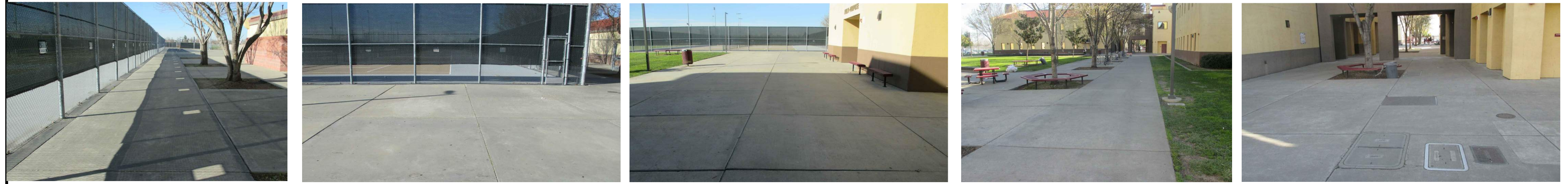
EXISTING CONDITION OF FUTURE GAS TRENCH. SAW CUT AT CONCRETE JOINTS. REFER TO DEMOLITION NOTES
